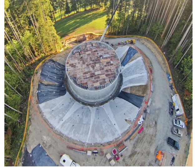
LOTT Reclaimed Water Tank L1200005
